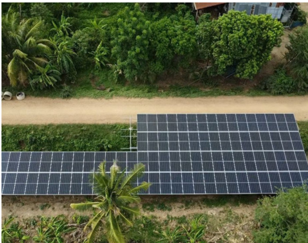
The solar panels installed in Peam village, Kdol Tahean commune, Bavel district ©EGE Cambodia
