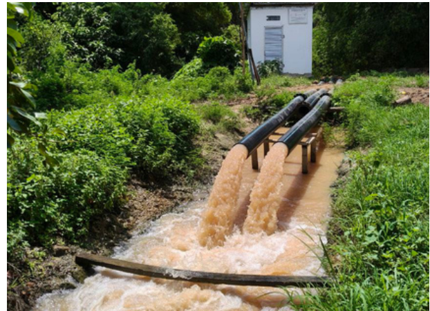
Solar pumping station supplying irrigation from the mainstream to sub-canals, Peam Village, Kdol Taken Commune, Bavel District, 2023. © EGE Cambodia
