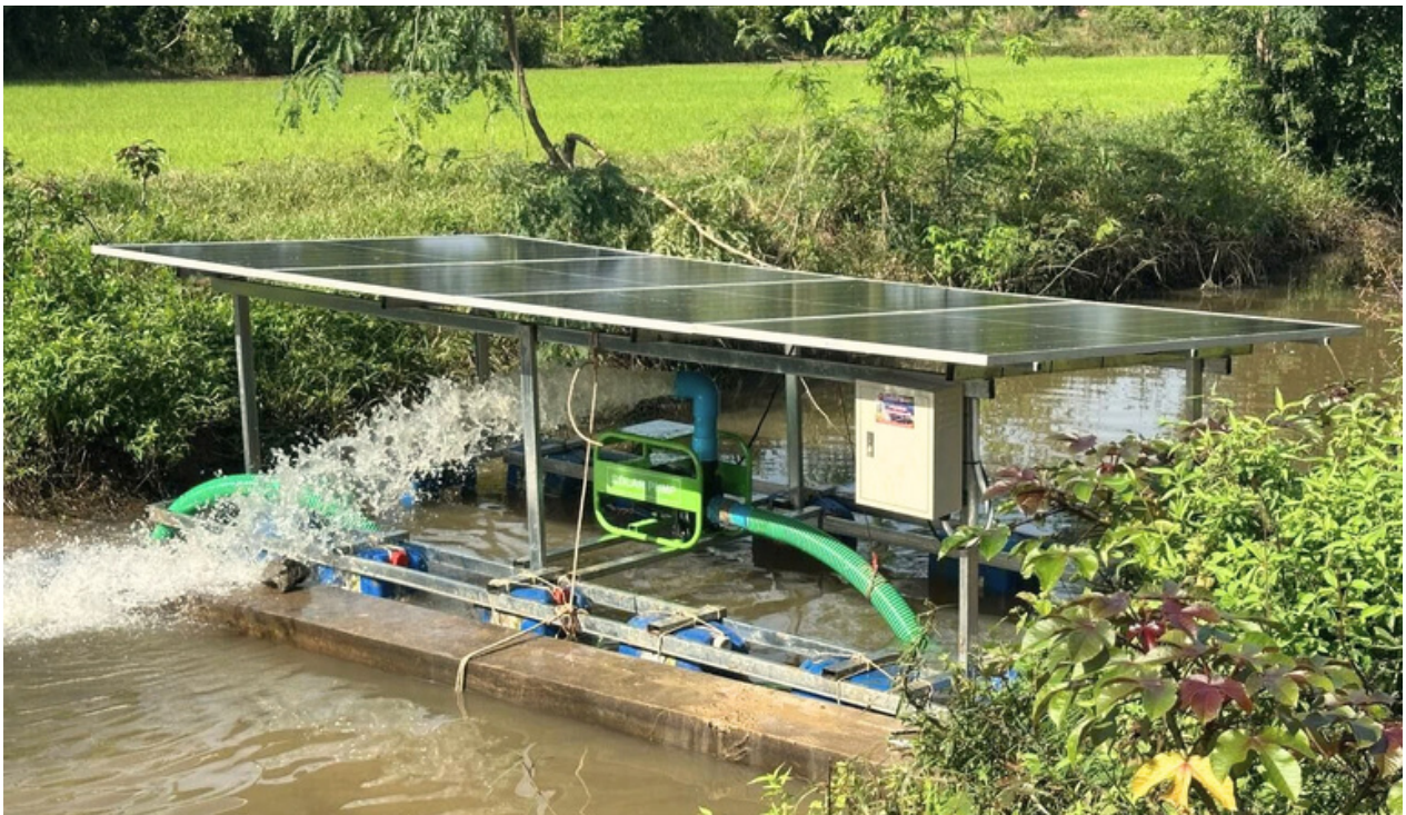
Floating pumping solar system in Peam village, Kdol Taken commune, Bavel district, 2023 ©EGE Cambodia
